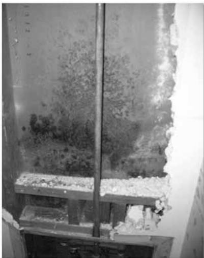
Figure 3. Mold growing inside a wall cavity on the back of drywall.
